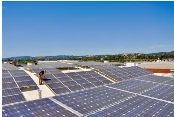
Scandic's solar panel array.
