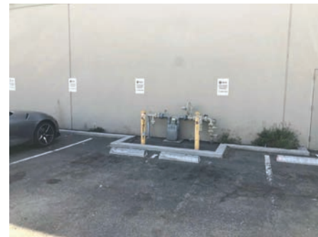
⑧ GAS METER
