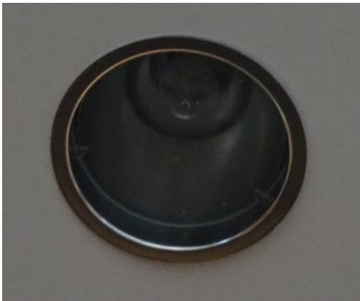
Existing Interior Lighting
