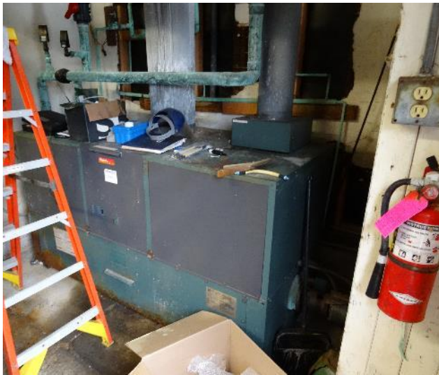
Existing Pool Boiler
