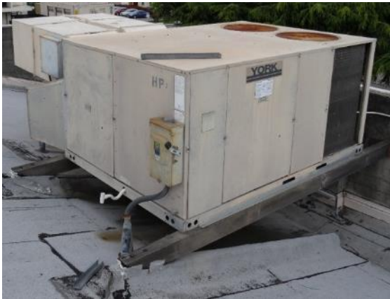
Existing HVAC Equipment
