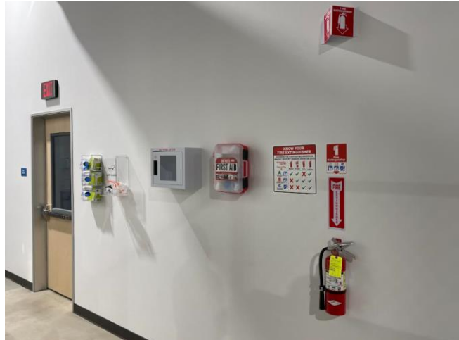
Figure 6 - A hallway with PPE, first aid kit, and fire extinguisher
