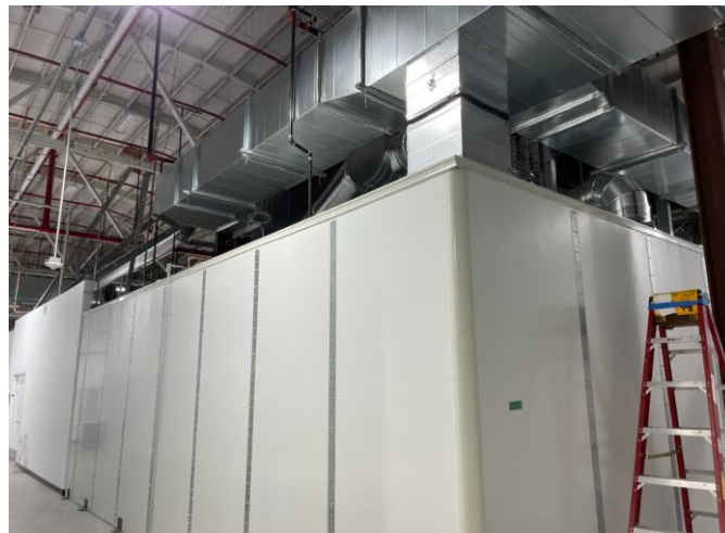
Figure 5 - Dry room exterior with duct work showing
