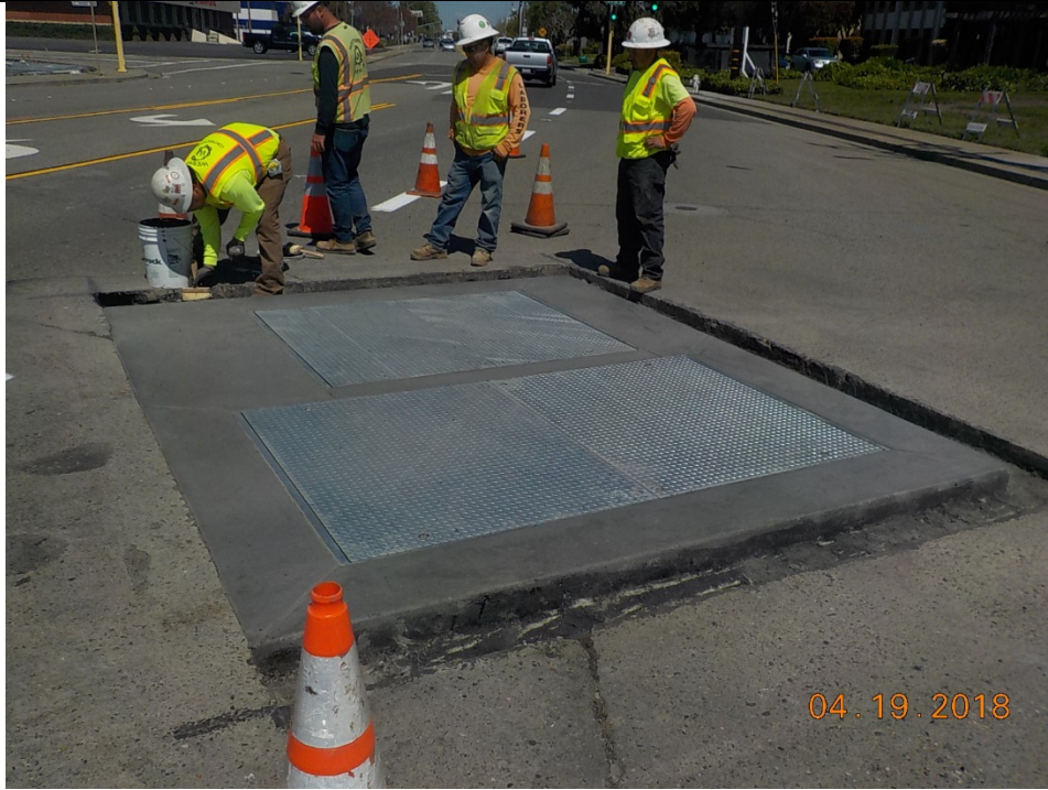
HEAVY TRAFFIC RATED VAULTS AT WICKS BLVD. /MERCED STREET
