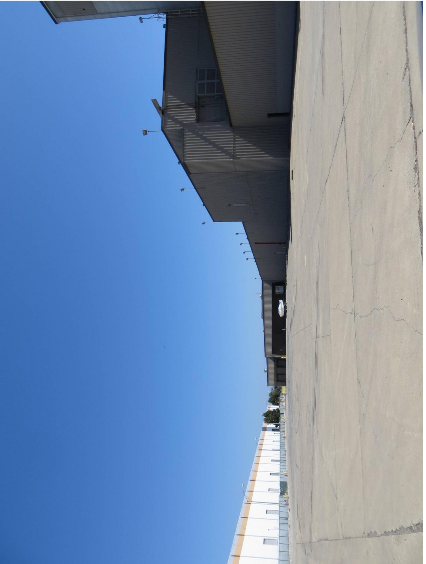
Figure 20. A View of the rear of the Kellogg Plant today - the inaccessible interior of a superblock.
