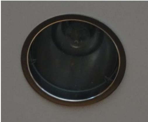
Existing Interior Lighting
