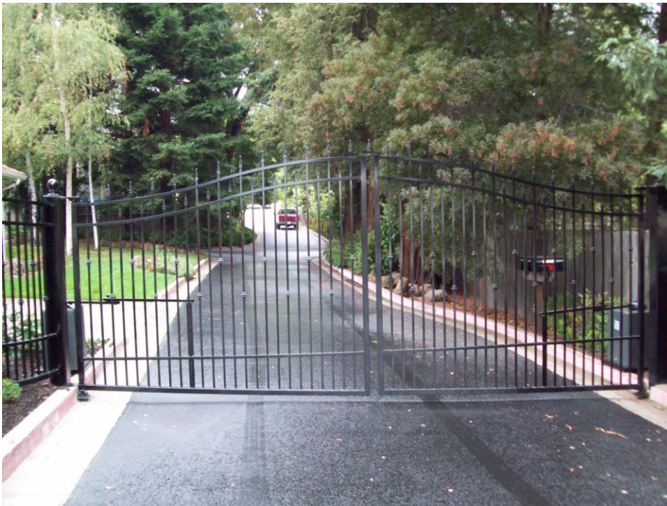
Photograph of Arched Tops for the Gates and the Twisted Knot Detail on the Vertical Bars at Floresta Gardens.
