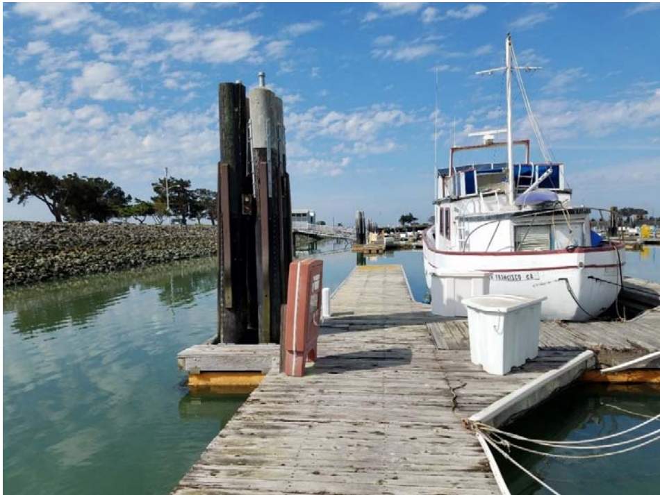
Photo 4 - Typical timber dolphin and floating dock. Note fiberglass jacket and concrete cap on the piles.
