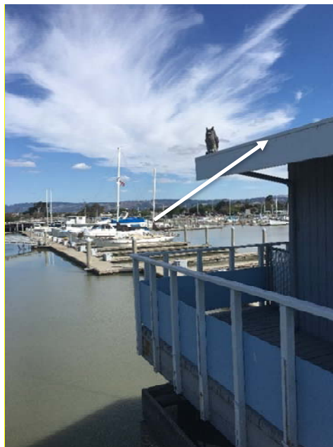
Photograph 7 – Marina – Harbor Master’s Office – Flashing and sealant (grey) (typical, indicated by white arrow) and reported contain asbestos.
