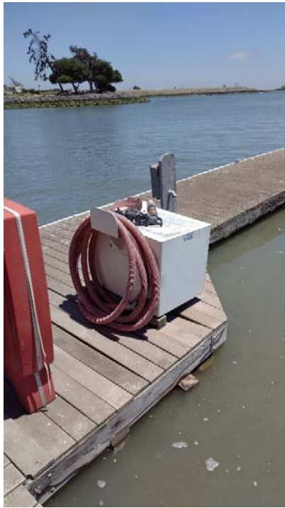
Photo 11 - Sewage Pump on Refueling Dock (typical of 2)
