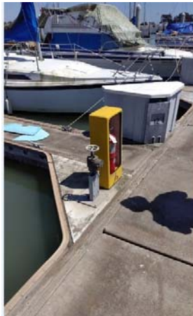
Photo 16 - Typical Fire Extinguisher and Hydrant
