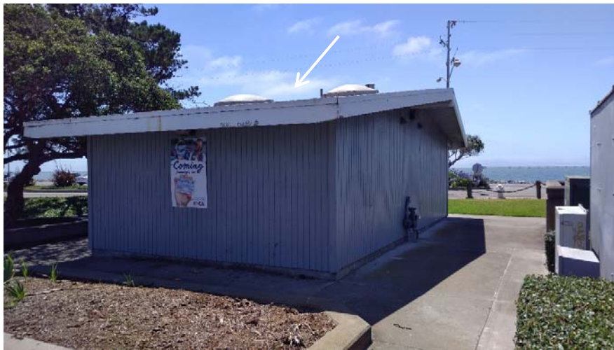
Photograph 1 – Marina – Restroom A, B – Roof penetrations – Penetrations throughout (indicated by white arrow) reported to contain asbestos.
