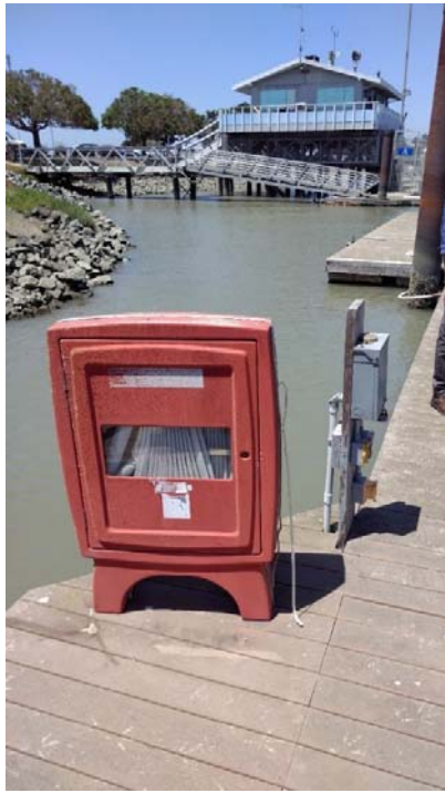
Photo 17 - Typical Fire Hose Cabinet
