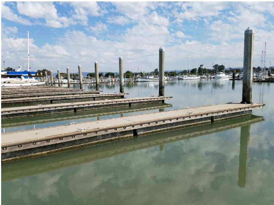
Photo 2 - Pier A -- Typical Concrete Float Condition
