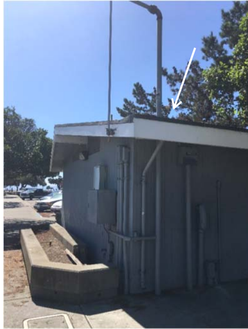
Photograph 6 – Marina – Restroom F – Roof – Roof Caulk (white/grey) (typical, indicated by white arrow) at penetrations throughout reported to contain asbestos.
