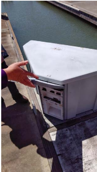
Photo 12 - Typical Service Cabinet – containing electrical, telecomm, and water service
