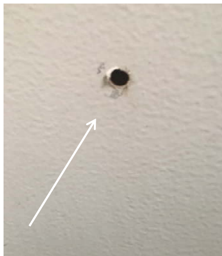
Photograph 2 – Marina – Restroom E, F – Wall texture (white) – Sampled at wall systems (indicated by white arrow) reported to contain asbestos.
