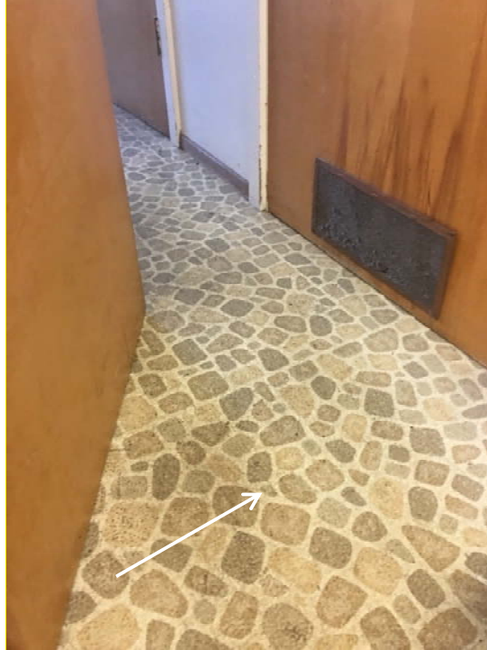
Photograph 4 – Marina – Harbor Master’s Office – Resilient sheet flooring (tan/gold), 12”x12” vinyl floor tile (not shown, located underneath RSF) (indicated by white arrow) both reported to contain asbestos.
