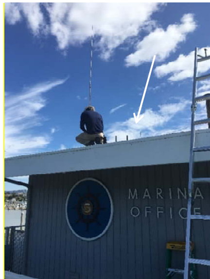
Photograph 5 – Marina – Harbor Master’s Office – Roof – Roof Penetrations throughout (grey and black) (typical, indicated by white arrow) reported to contain asbestos.
