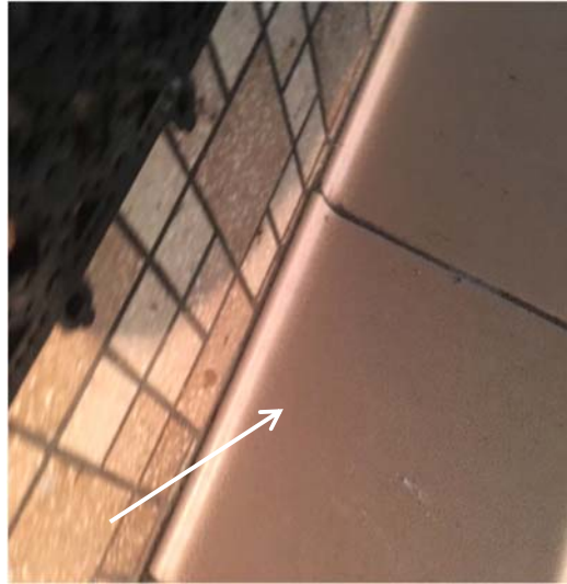
Photograph 3 – Marina – Restrooms E interior – Ceramic tile mastic (tan) located underneath tile - associated with floor and wall systems (indicated by white arrow) reported to contain asbestos.
