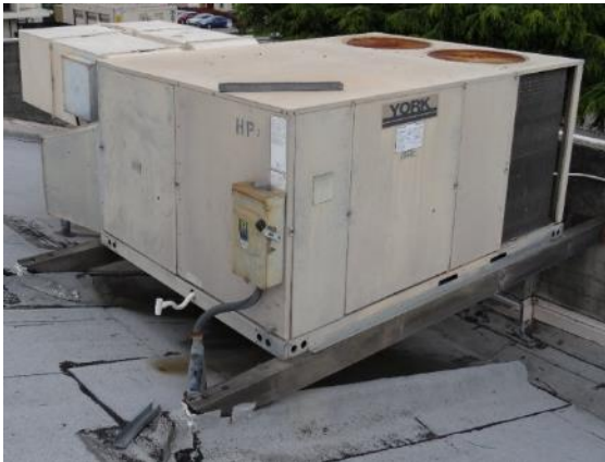
Existing HVAC Equipment
