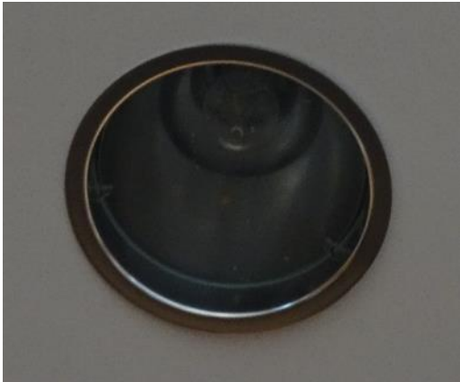
Existing Interior Lighting
