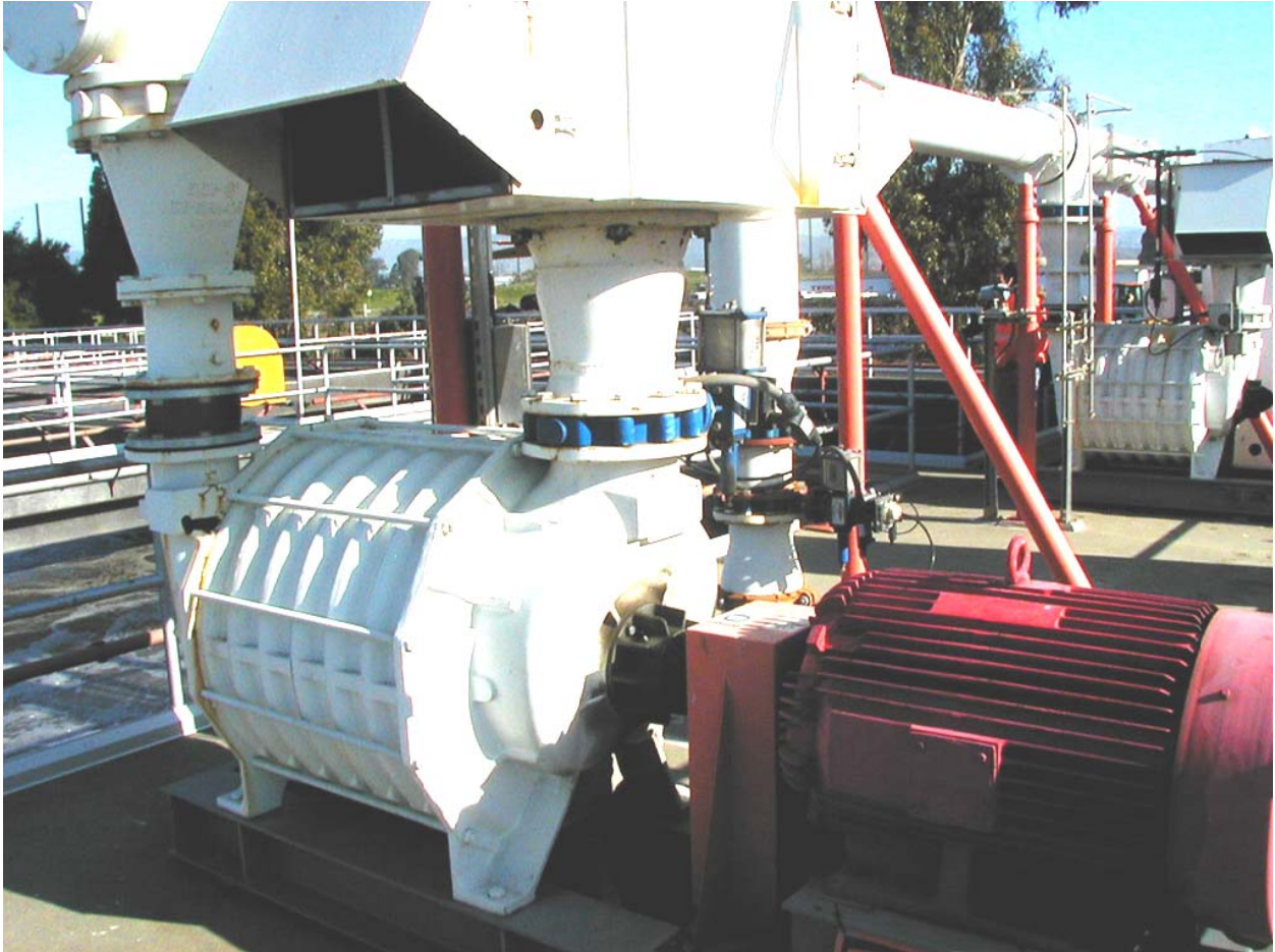
Figure 2.1.1.1 – San Leandro Multistage Aeration Blowers
