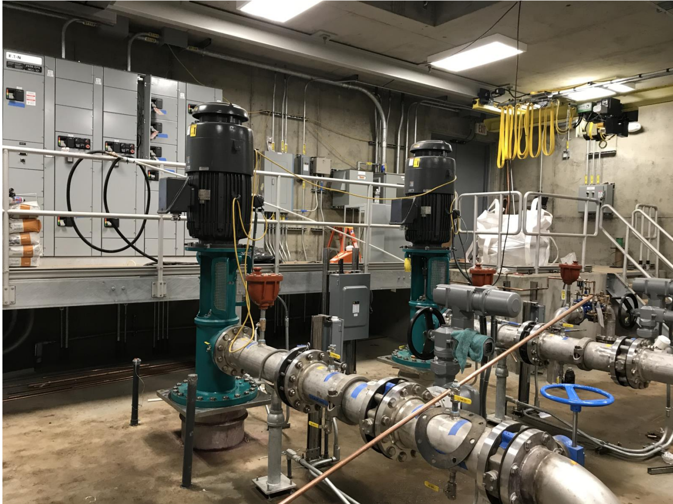
Bayfair Pumping Plant
