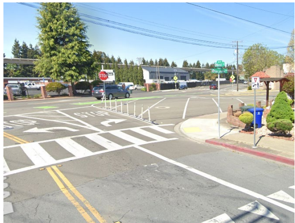
New curb extension to narrow the intersection, including accessible ramps and high-visibility crosswalks at San Leandro Boulevard and Best Avenue.
