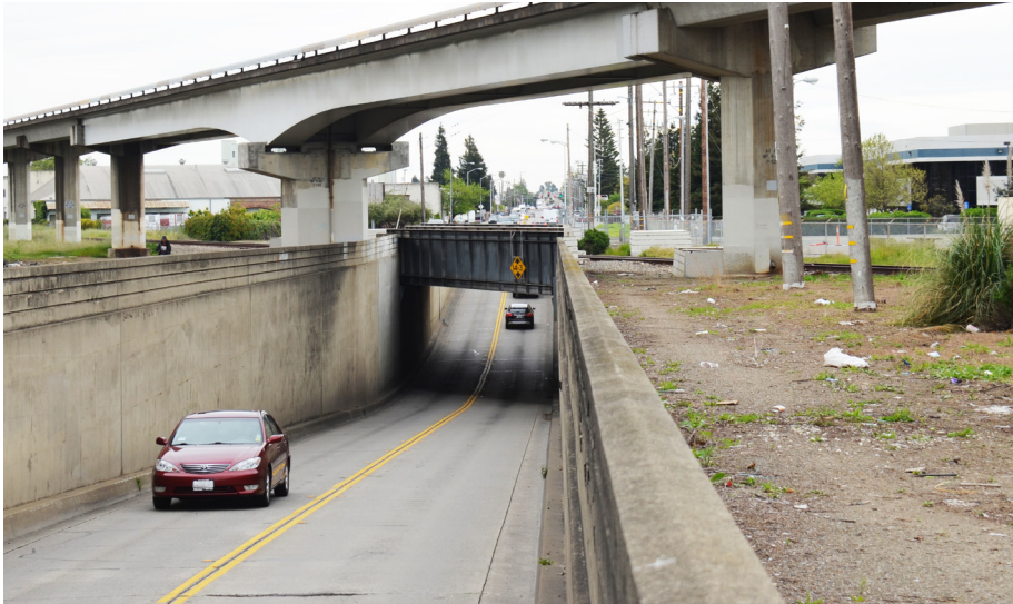
The Washington Avenue tunnel and adjacent area. The at-grade Union Pacific tracks are in the background under the above-grade BART tracks.
