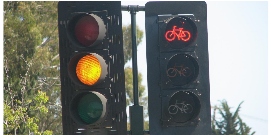
A bike signal mounted next to a standard signal in San Luis Obispo.
