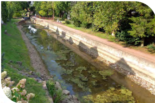
Storm water canals
