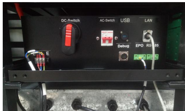
Figure 8 String control tray
