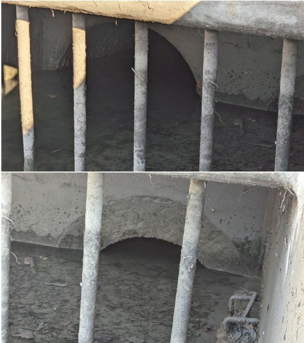
Figure 3-6: Heavy Blockage in 66-inch (top) and 48-inch (bottom) Pipes at Low Tide
