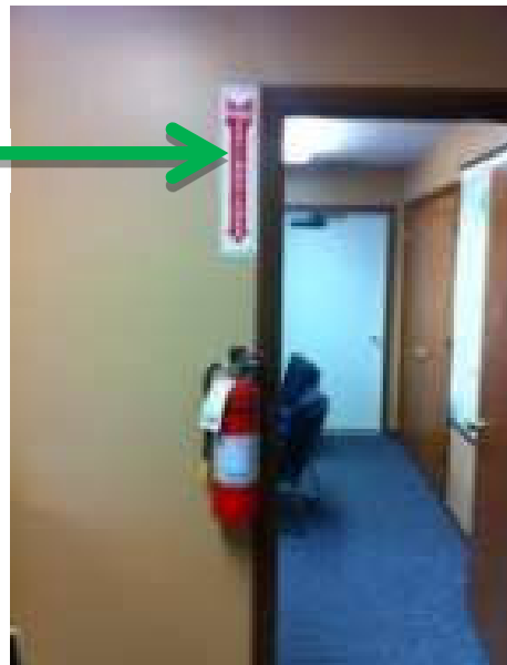
Fire Extinguisher Sign
